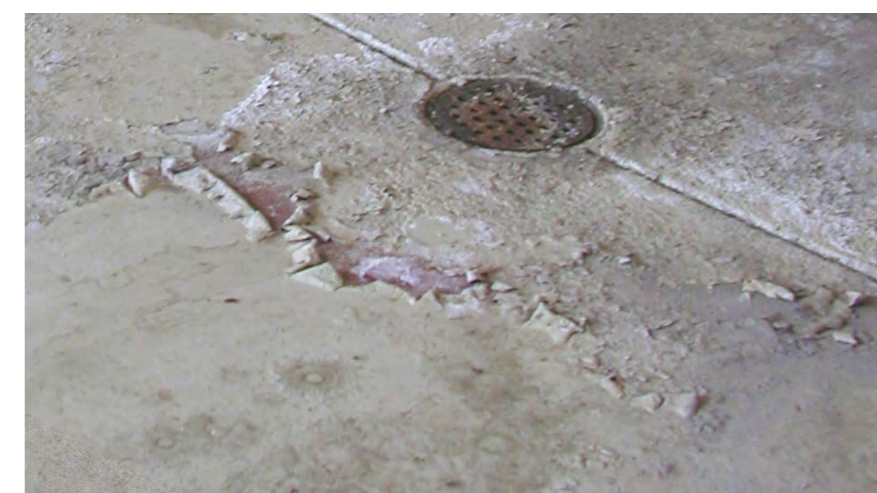
Moisture gets trapped under sealed or painted concrete, causing peeling
