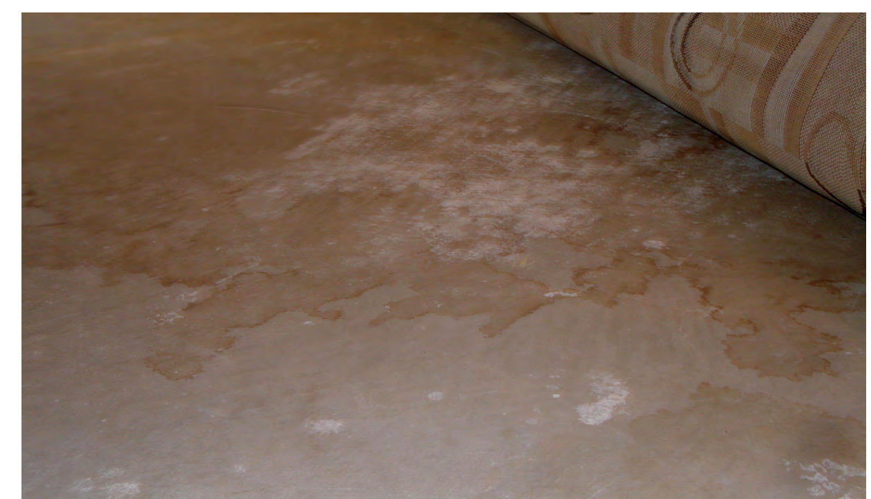
Mold under carpeting caused by moisture and no air circulation
