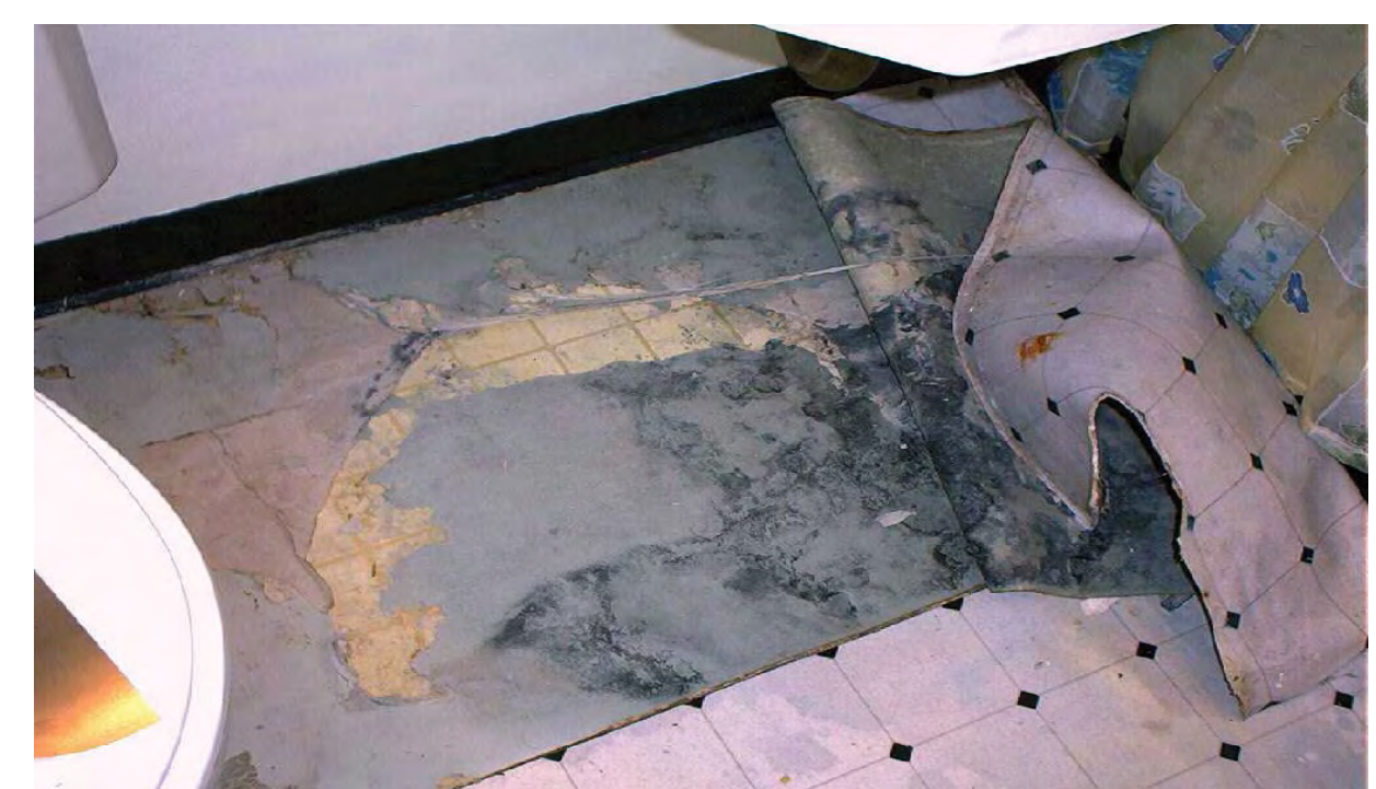
Mildew under linoleum as a result of moisture and no air circulation
