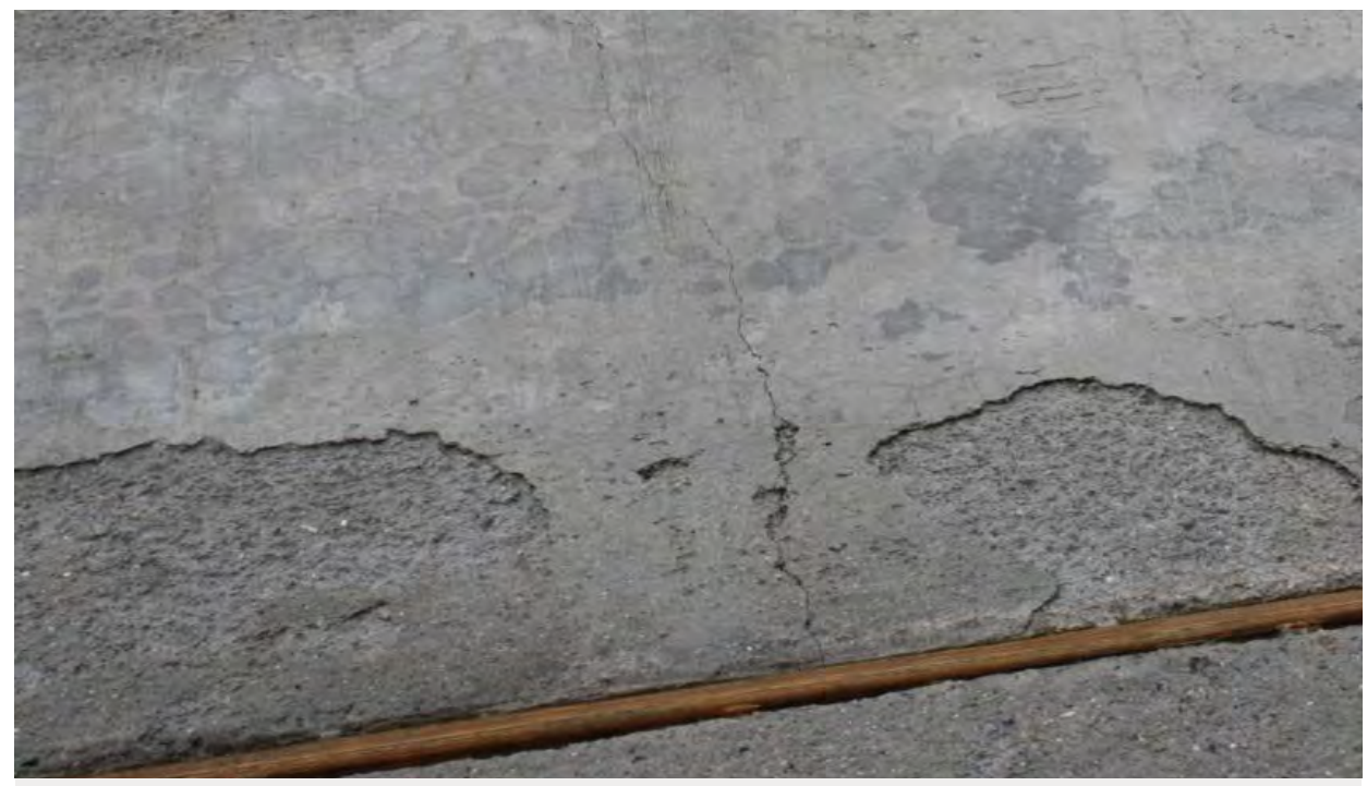
Moisture in concrete can cause ugly spalling or flaking and create a tripping hazard
