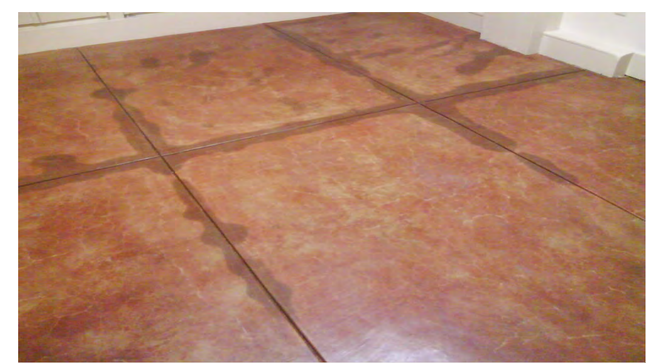
Moisture seeps through tile, promoting the growth of mold and mildew
