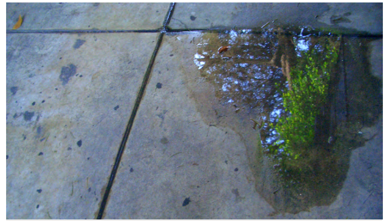
Water can pool on uneven concrete, which is can cause spalling over the long term
