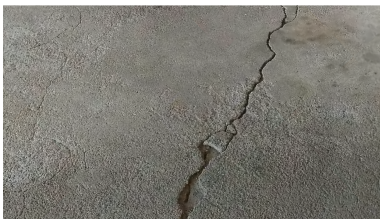
Unsightly cracks caused by the freeze/thaw cycle make your garage less welcoming
